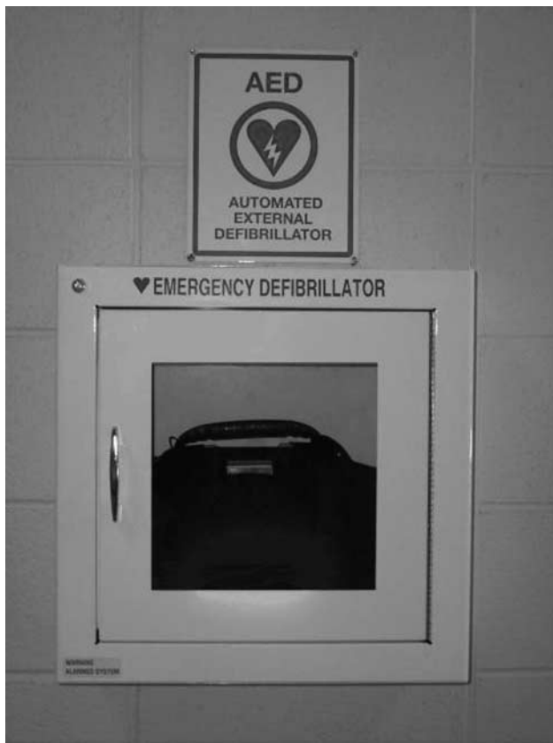
Figure 1 AED in wall-mounted storage cabinet.
