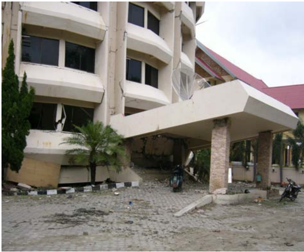
Fig. 1.15 Building after the first floor collapsed in the earthquake.
