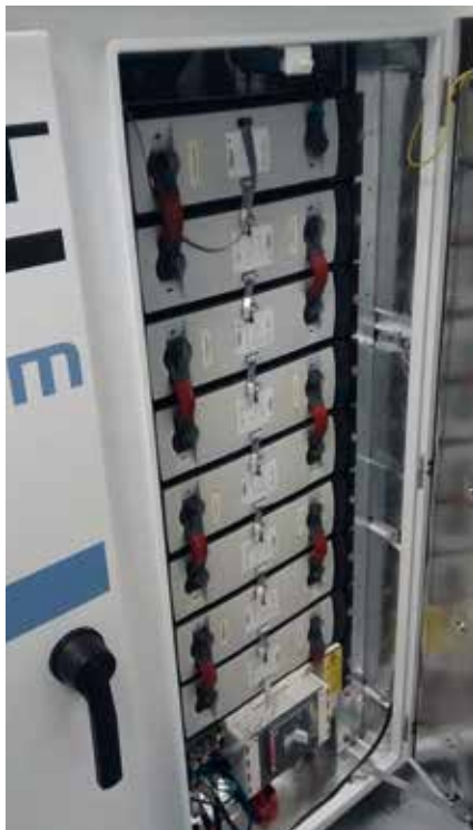
Figure 58 - Li-ion battery deployed in one demonstration case in Spain
