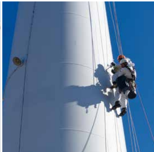
Figure 41 - Installation of an autonomous video-based bird monitoring and dissuasion system on the nacelle of a wind turbine at CRES demonstration wind farm, PENA (GR). The system detects/records movements of flying objects in the area, assesses them and makes decisions to trigger bird collision mitigation measures (sound emission, wind turbine stopping) in real time, depending on the risk of impact.
