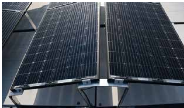
Figure 15 - BI-FACE bifacial modules with optimised design. A white painted ground helps to boost the reflected light to the rear side of the modules.
