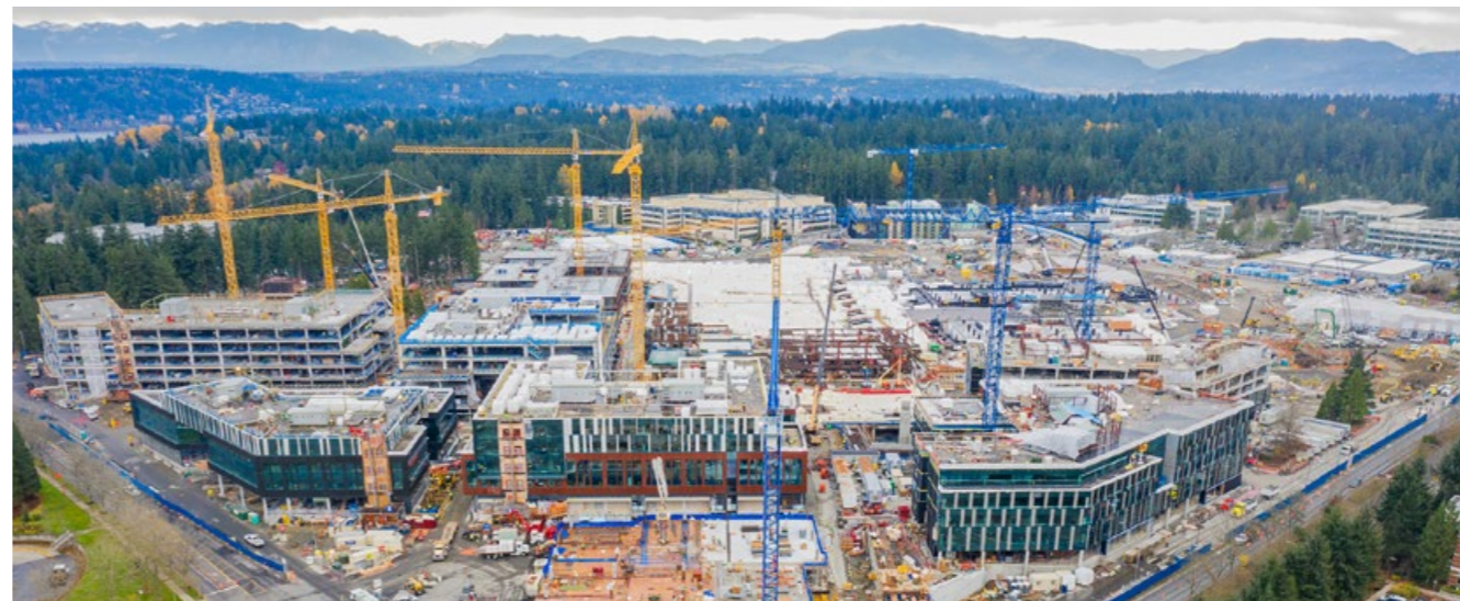
Our Puget Sound modernization project is currently achieving over 90 percent construction waste diversion.
