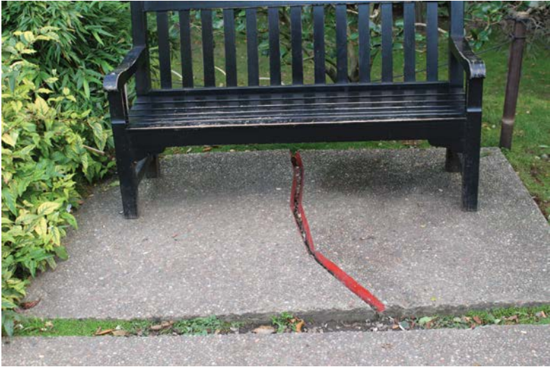
Fig. 9.6 The crack under the bench in the Kyoto Garden. Source: author
