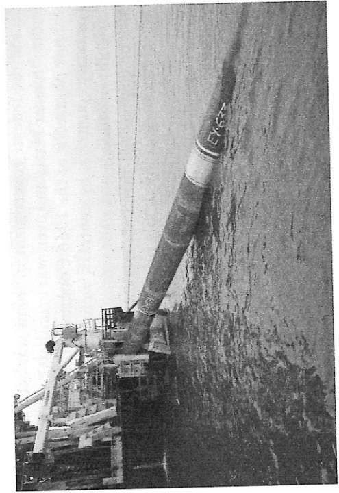
Figure 6.2 Constructing the Nord Stream I pipeline. Poland’s foreign minister Radosław Sikorski famously dubbed Nord Stream the “Molotov-Ribbentrop Pipeline”, and other actors criticized the project on environmental grounds. Here the pipeline is being lowered into the Baltic Sea by the Italian vessel Castoro Dieci in summer 2011. Photo: Nord Stream AG.
