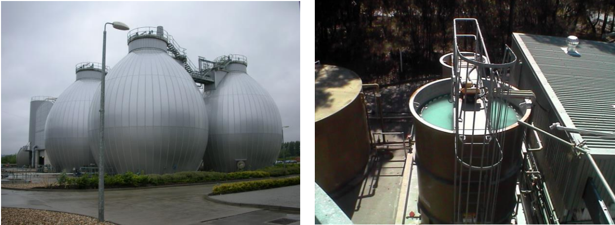
Figure 2: Photographic examples of closed systems: biodigestors at a sewerage treatment plant in Reading, United Kingdom (left); industrial wastewater bio-chemical treatment plant in Brisbane, Australia (right).
