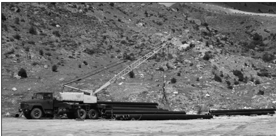
Fig. 5. Unloading of pipe in North Ossetia for construction of the Alagir–Tskhinvali natural gas pipeline. Photograph by the author, August 2007.
