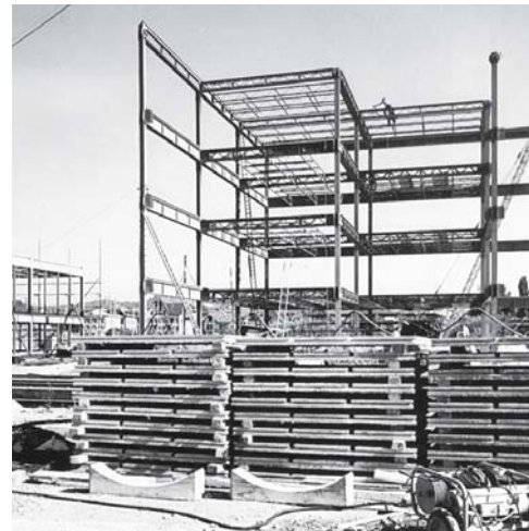
Fig. 113: Steel frame with beams at the same level, floor bays as subsystem Fritz Haller: canton school, Baden (CH), 1962–64
