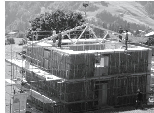
4 Structural shell almost complete, only the protective layer of render has yet to be applied
