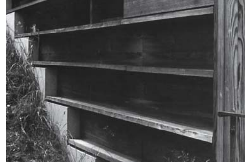
Fig. 68: The concrete plinth is the visible part of the excavation in which this timber building stands. Horizontal boards positioned at the steps in the concrete cover the concrete/timber junctions. Peter Zumthor: Gugelun House, Versam (CH), 1994
