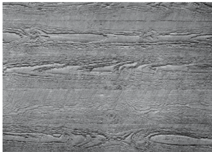
Fig. 24: Horizontal timber boards Formwork made from 3 cm thick Douglas fir boards, straight edges, butt joints between boards.
