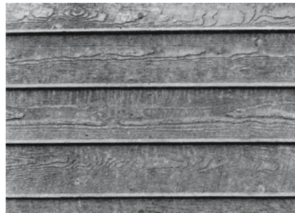
Fig. 25: Horizontal timber boards Formwork made from 18 cm wide, 3 cm thick Douglas fir boards, chamfered edges, tight butt joints between boards. Characteristic, projecting concrete fins are the result.
