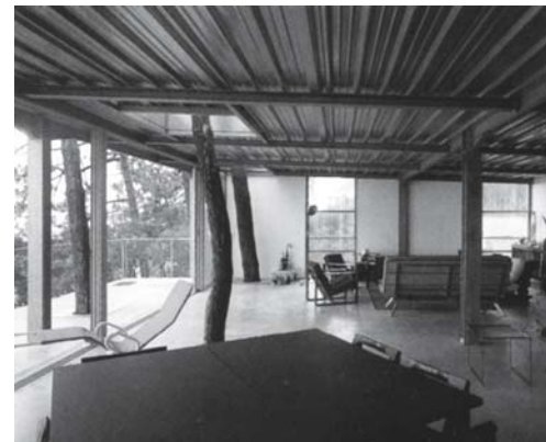
Fig. 60: Steel frame and corrugated sheets left exposed internally Lacaton & Vassal: holiday chalet, Lège Cap-Ferret (F), 1998
