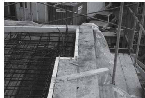
Fig. 51: Close-up of formwork The slab edge elements act as a permanent formwork; gypsum boards provide a space for the insulation.
