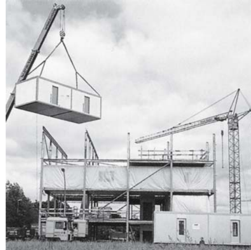
Fig. 126: Container (e.g. as meeting room) supported on steel frame Dollmann + Partner: office building, Fellbach (D), 1999
