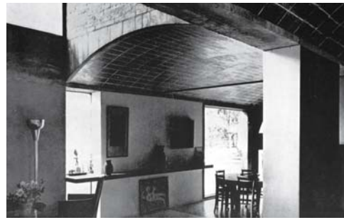
Fig. 39: Brickwork vaulting as permanent formwork to concrete above, with tie bars to accommodate thrust. The vaulted construction here has an architectural, space-forming value.
