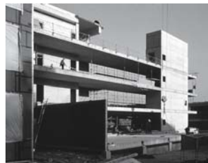
Fig. 267: Concrete cores Under construction, 1997; the concrete floors support only their own self-weight and therefore large spans and cantilevers are possible.
