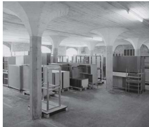
Abb. 63: Flared column heads transfer the loads from the upper floors into the columns.
