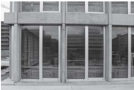
Fig. 226: Facade to secondary school Window with fixed light and bottom-hung light, fixed desks and radiators
