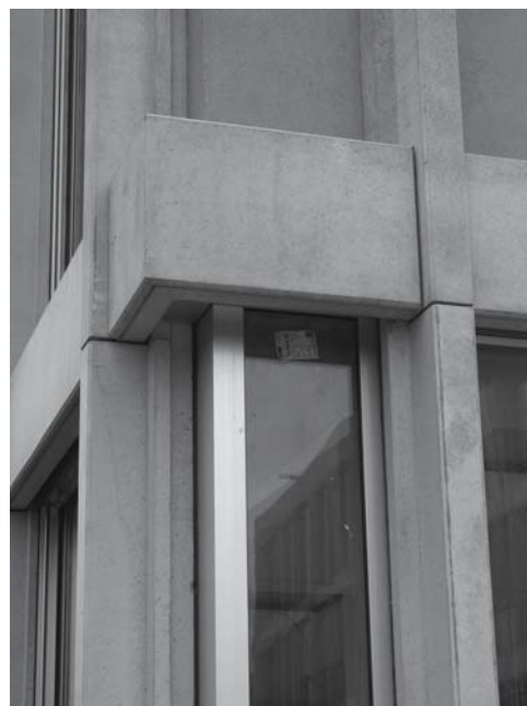
Fig. 229: Close-up of facade Corner between ground and 1st floor levels on primary school building
