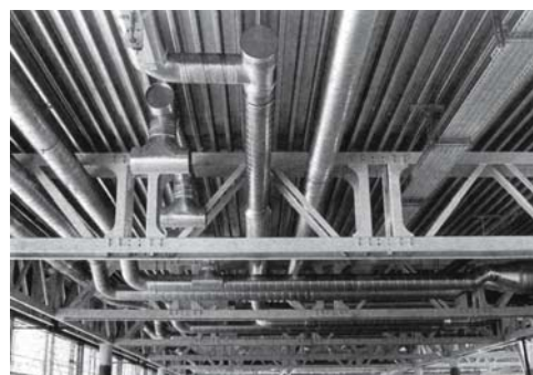
Fig. 10: Services in the plane of the loadbearing structure Fritz Haller: SBB Löwenberg Training Centre, Murten (CH), 1980–82
