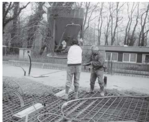
Fig. 3: Prior to pouring the concrete: formwork, reinforcement and any services (electric cables, water pipes, ventilation ducts, etc.) that are to be cast in
