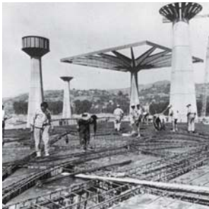
Fig. 76a: Canopies under construction Pier Luigi Nervi: Hall of Labour, Turin (I), 1961
