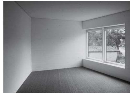
Fig. 304: Internal view of window on 2nd floor The reveal merges into the wall.
