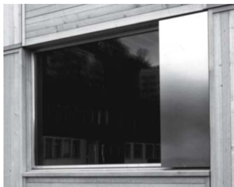
Fig. 281: Sunshading Sunshading in the form of an aluminium shutter in front of the ventilation light plus a fabric awning in front of the fixed light
