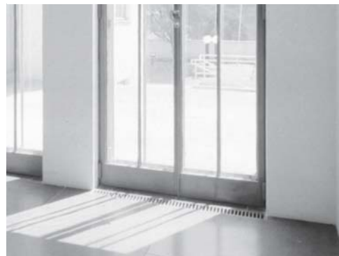
Fig. 17: Underfloor heating plus hot-air ducts supplied from the cellar (in front of French windows) Ludwig Wittgenstein: house in Kundmannngasse, Vienna (A), 1928
