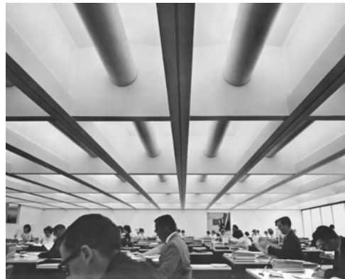
Fig. 27: Floor slab without intervening columns, with ventilation ducts and lighting units between the ribs SOM: American Republic Insurance Company, Des Moines (Iowa, USA), 1965
