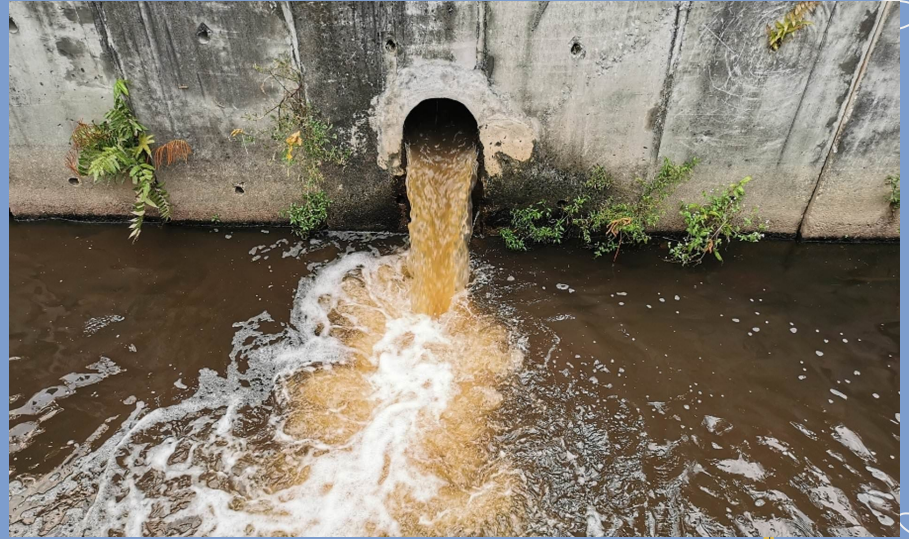
Sewage water leak
