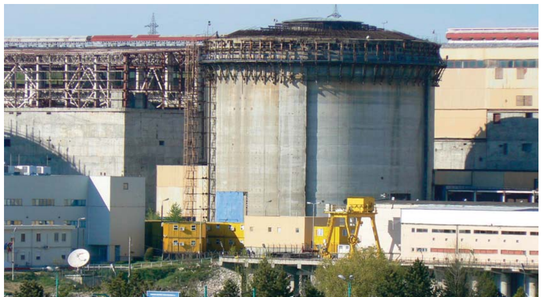
The second reactor at Cernavoda nuclear power plant close to completion in 2007, and now in operation. The other three reactor buildings are degrading.
