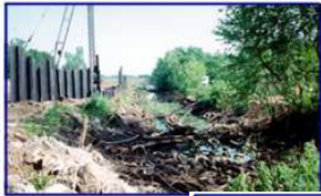
The East Ditch, located at the sou contained discarded tires and deb
