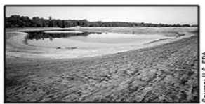
1993: After excavating soil, the wet field was graded and seeded to support wetlands. Source: U.S. EPA
