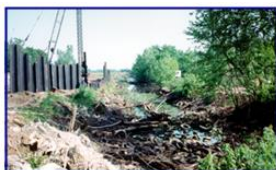
The East Ditch, located at the source, contained discarded tires and debris.
