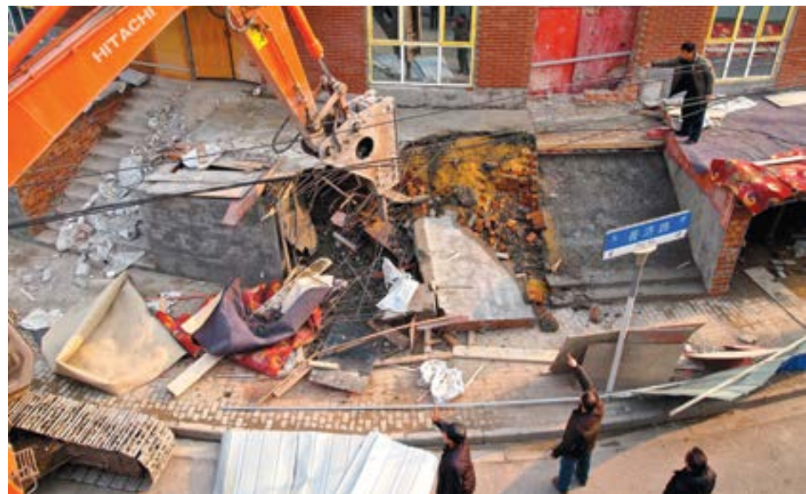
Three people give directions to a bulldozer driver demolishing an illegal structure, Shanghai, 29 January 2013. Photo: Remko Tanis
