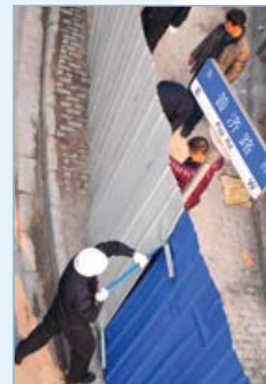
Chengguan officers busy taking down the fence around an illegal construction before demolition, while being filmed by local TV, in Zhabei district, Shanghai, 29 January 2013. Photo: Remko Tanis
