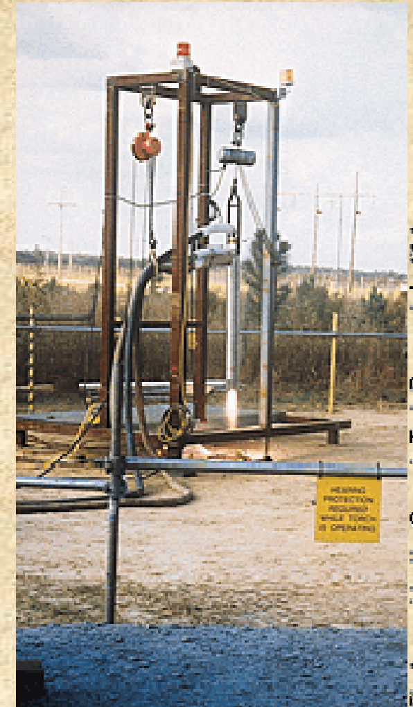
Plasma torch suspended above borehole prior to the Savannah River Site demonstration.
