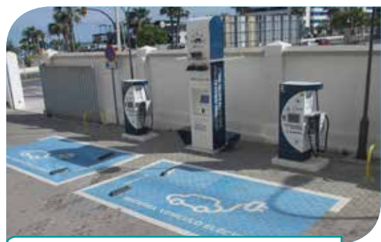
Charging stations in Malaga, © Malaga City Council
