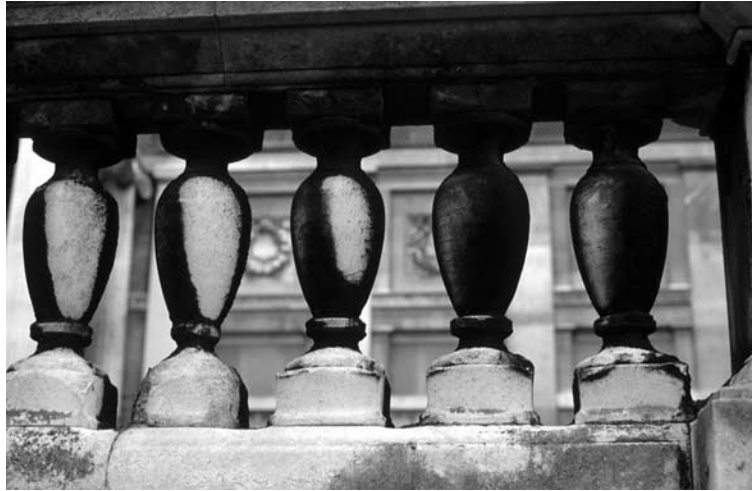
Plate 6.4 Weathered balustrade on the Ashmolean Museum, Oxford, England. The balustrade has now been cleaned. ( Photograph by Heather A. Viles )
