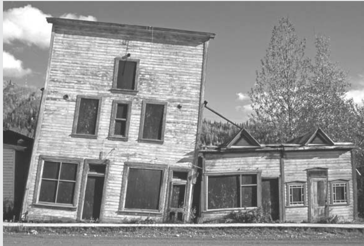
Plate 11.9 Subsidence due to thawing of permafrost, Dawson, Klondike, Alaska, USA. ( Photograph by Tony Waltham Geophotos )
