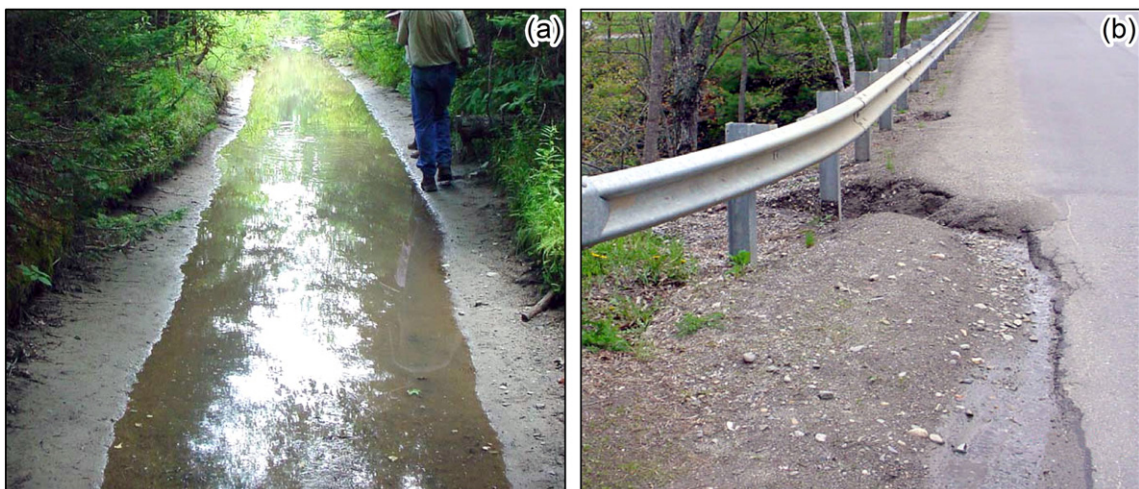
Fig. 10. Road effects on streams and erosion. (a) Off-highway trail capturing a local stream. (b) Sand building up at a road crossing and washing down into the West Branch of the Sheepscot River, as indicated by the gully between the third and fourth guard rails (Klamath Resource Information System—KRIS, 2015).
