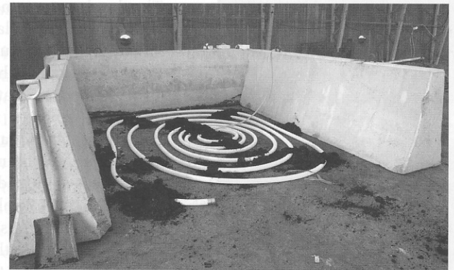
Fig. 22.6. Spiral aeration system of a fungal pilot pile. It can be connected to a compressor for continuous active aeration
