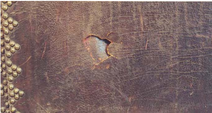
Figure 23.23 Damage before repair using low pressure suction box.
