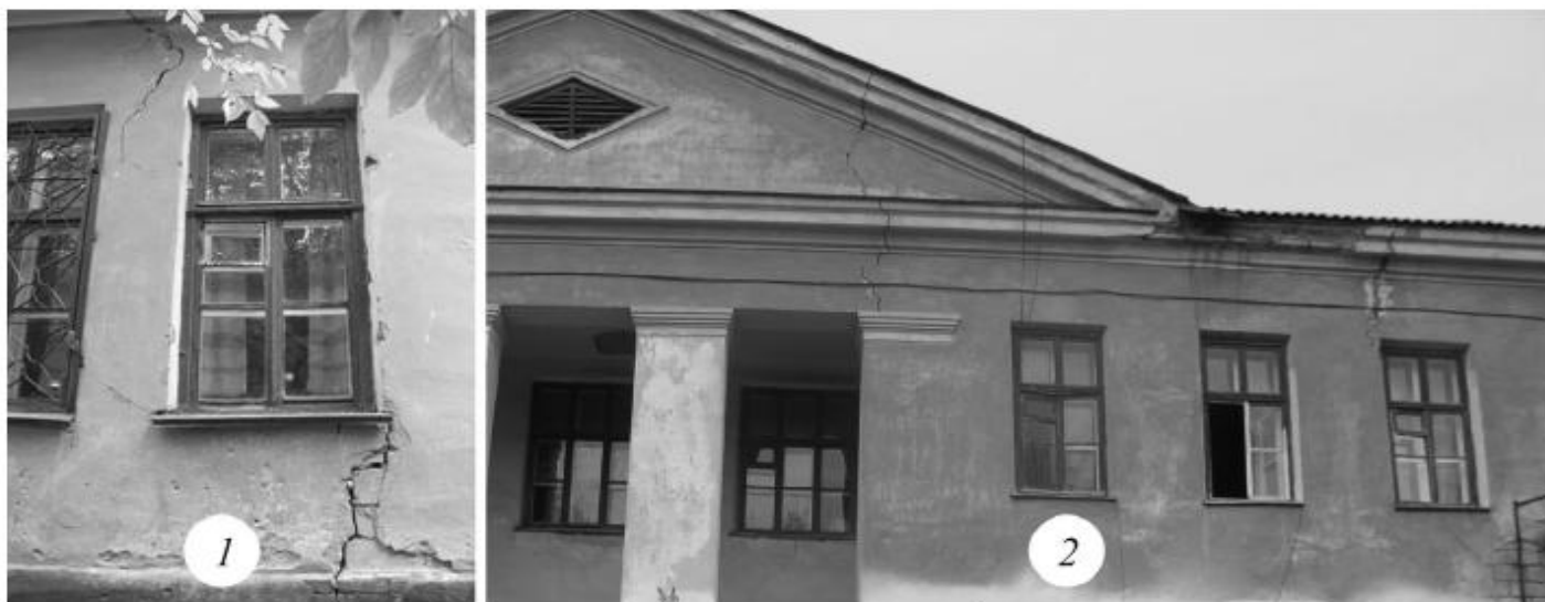
Fig. 1. Structural damage of a building front: 1—cracking, side wing, ground floor; 2—damage in the central part, first floor.
