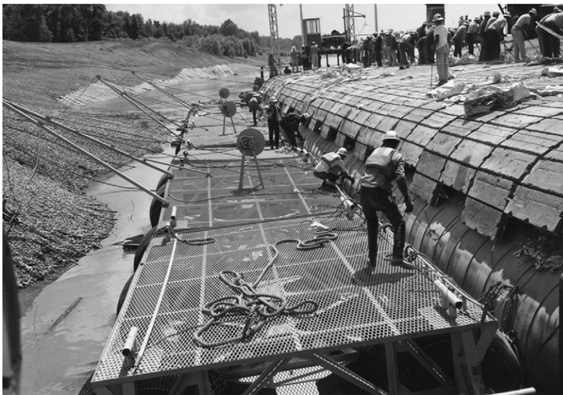
Fig. 9. Construction of articulated concrete revetment for bank protection (1964) at Goldbottom, Mississippi (photo: US-ACE).
