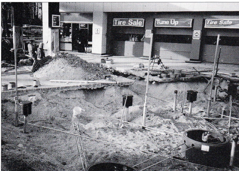
FIGURE 18.2 Leaking underground storage tank (LUST) replacement at a gas station in California. The old rusting steel tanks have been removed and replaced by more corrosion-resistant fiberglass tanks, which are set in the ground and covered with pea gravel. The soil and groundwater aquifer beneath the tanks were cleaned up using special techniques to stimulate soil microorganisms and to pump out volatile organics such as benzene vapors. Remediation and replacement typically costs $500,000 for a single gas station. (Photo courtesy of R. Weil)
