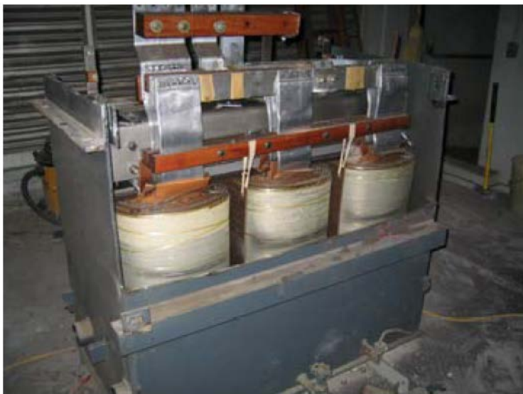
Too big to be taken down elevator
