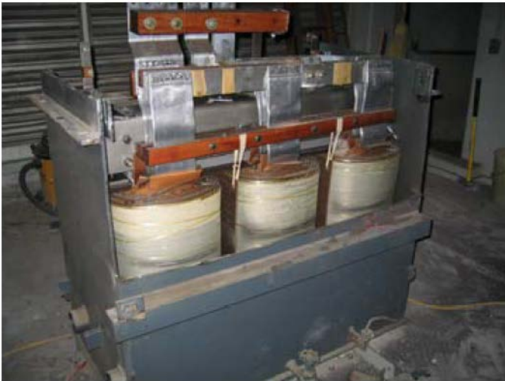
Too big to be taken down elevator
