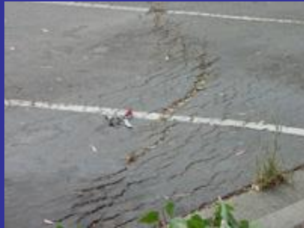
Contra Costa, deformed road
