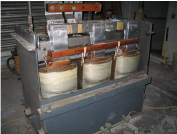
Too big to be taken down elevator
