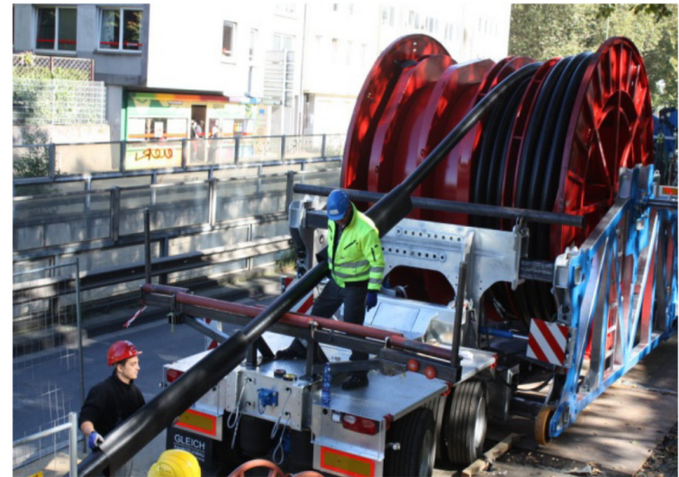
Fig. 6. Pulling of the first cable length from the joint bay to substation Dellbrügge.
